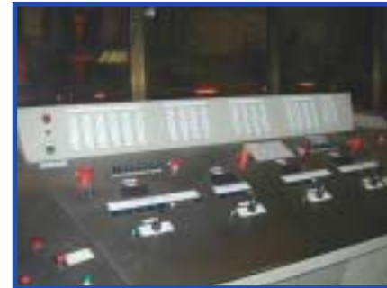
Main Control Pulpit
