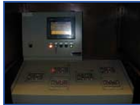
Local Control Panel
